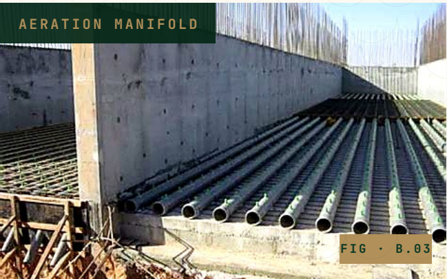
HDPE aeration manifold beneath each bay, zoned for Phase-I.
