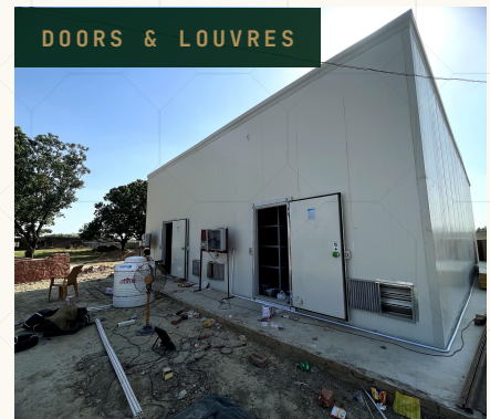
PUF access, exhaust stacks
